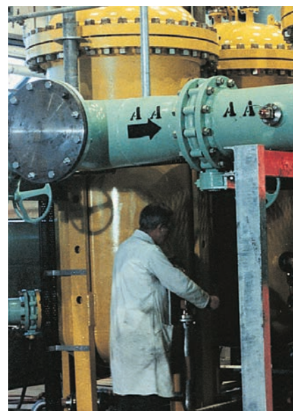
Pall's blowback filter system in operation.
